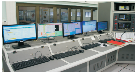
Fig. T.1.6: Main control system at ARPF for monitoring and regulating linac and process operations.
