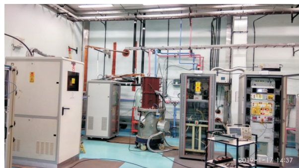
Fig. T.1.5: Microwave system for linacs
