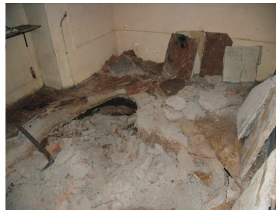
Fig. I.2.2: Damaged hollow floor.
