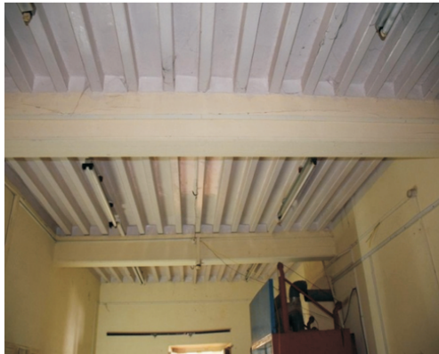
Fig. I.2.4: Deflection of wooden beams.
