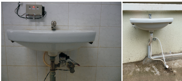
IR sensor based and foot-operated wash basins.
