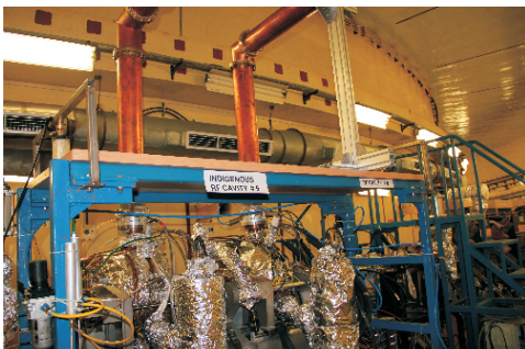
Fig. T.1.6: 505.8 MHz OFE copper RF cavity installed in Indus-2.
