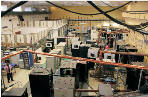
Fig. T.1.5: High power SSPA installed in Indus-2.
