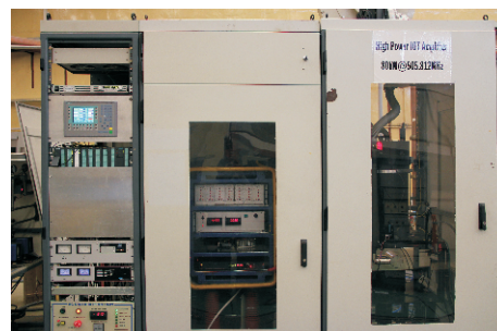
Fig. T.1.4: 60 kW IOT amplifier at 505.8 MHz.
