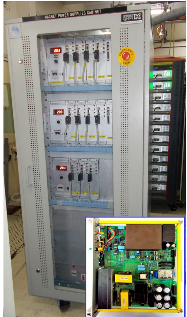
Fig. A.4.1: A photograph showing newly installed power converters for steering coils in TL-2. The inset shows one power converter card.
