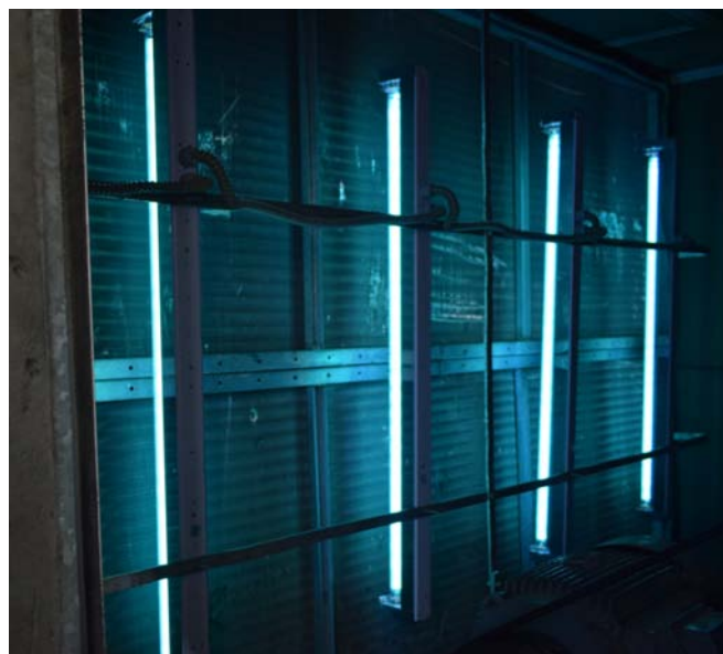
Fig. I.2.2: Photograph showing germicidal UV-C lamps integrated in AHU at Indus-2 complex.
