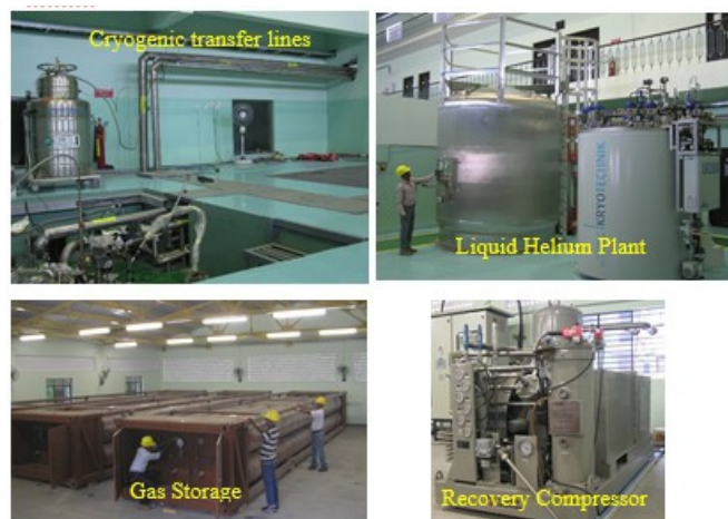
Fig T.1.16: Cryogenic facilities for cavity test stands.
