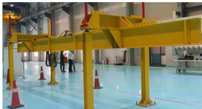
Fig. T.1.25: Lifting tool installed at New Cryomodule Building will be used as first assembly station of 650 MHz cryomodule.
