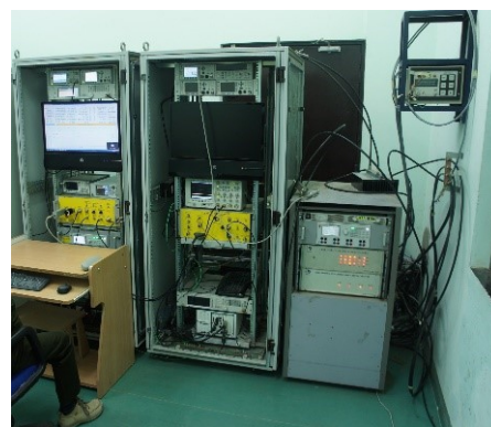
Fig. T.1.17: VTS control room during cavity test.
