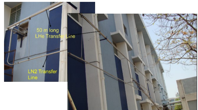
Fig. T.1.20: Cryogenic transfer lines for HTS.
