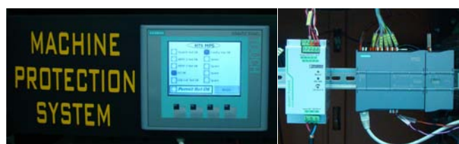
Fig. T.1.23: PLC based Machine Protection System.
