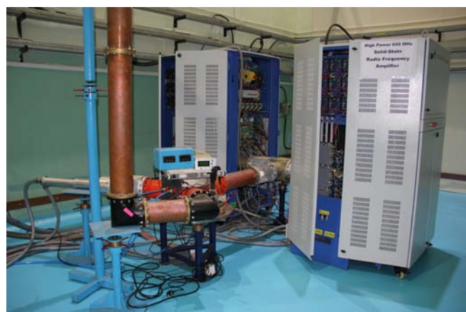
Fig. T.1.24: 32 kW RF SSPA along with circulator.
