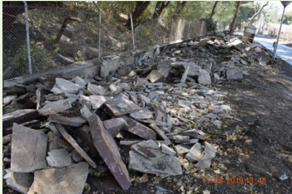
Fig. 30 Debris collected at construction sites (1/2)
