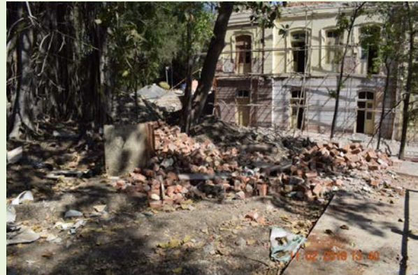
Fig. 31 Debris collected at construction sites (2/2)
