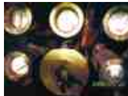
Fig.T.3.6: A site view of laser based bellow lip cutting in NAPS#1 reactor.
