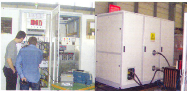
Fig. A.12.1: Inspection and evaluation testing of the modulator on a 110 kV load at CERN Test Stand
