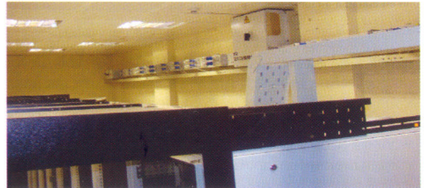
Fig. I.4.5 Luminaires & Bus Trunking System in Data Centre Hall of IT Extension Building
