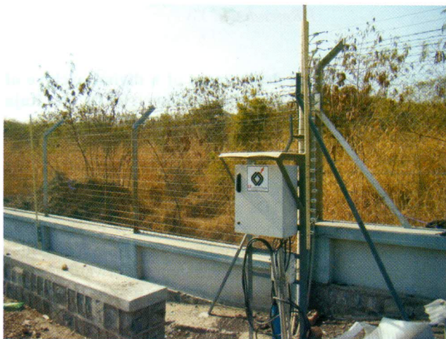
Figure I.5.1: A portion of electrical fence with an energizer
