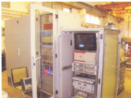
Fig A.6.1: 100kV Solid state bouncer modulator with PC based control system for 1MW Klystron TH 2089.
