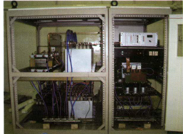
Fig. A.12.2: Photograph of the power source
