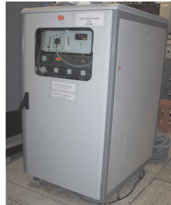
Fig. A.5.2: A photograph of the power supply installed in Indus-1 magnet power supply hall.
