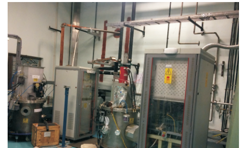
Fig. A.2.4: Microwave system and coolant distribution for both the linacs are seen in the Equipment Room of ARPF.
