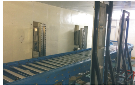
Fig. A.2.3: Process Chamber at ARPF. Two beam scanners, beam catchers and a segment of product handling system are seen.
