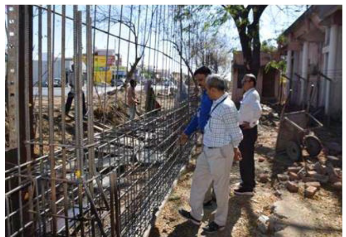
Team of judges inspecting the civil construction site for debris management and general cleanliness.
